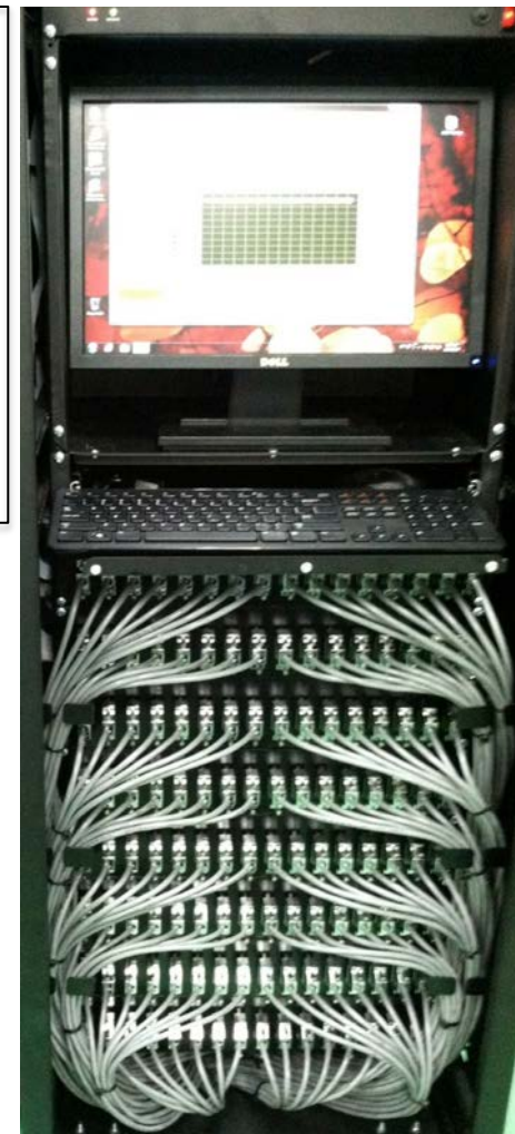
Electronics for 128 channel system at Mitsubishi Plastics, Inc.
