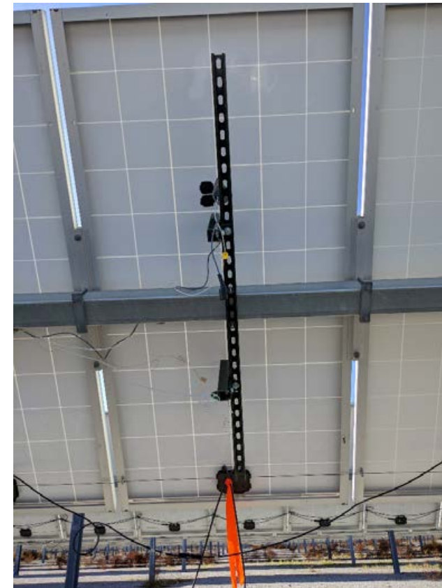
Installation of back of module sensors: two potentiometers along the centerline to measure displacement, an accelerometer to measure vibration, and a thermocouple
