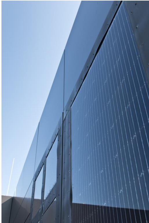
Building-integrated PV @ Energyville site
